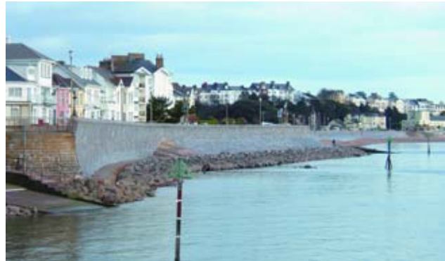
Image 7d: Foundations of the original sea wall at Exmouth revealed and reinforced with rock armour Source: Exe Estuary Management Partnership
