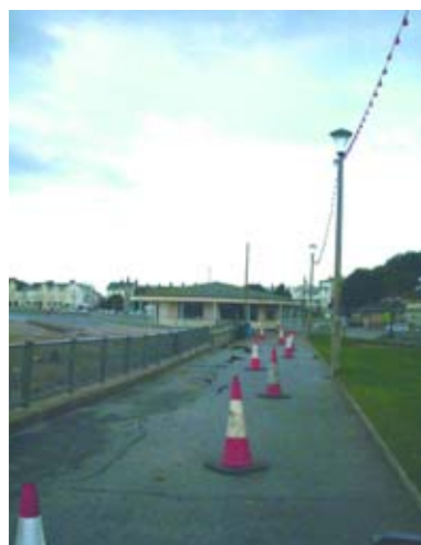
Image 7e: Sand lost from Exmouth after the storm October 2004, revealing foundations of the sea wall Source: Exe Estuary Management Partnership
