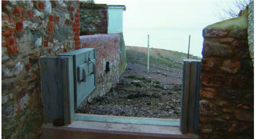
Image 7n: Flood gate as part of Lympstone's new tidal defence scheme Source: Exe Estuary Management Partnership
